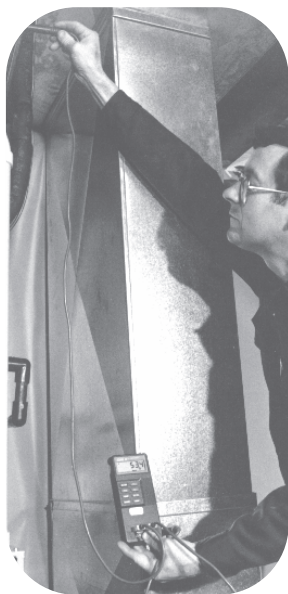
FIGURE 48 TEMPERATURE RISE MEASUREMENT
