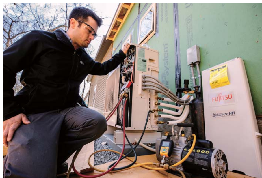
Dustin Ebersole, owner of High Efficiency Solutions, LLC, pulls a vacuum before starting the new multi-zone Fujitsu Halcyon unit.
