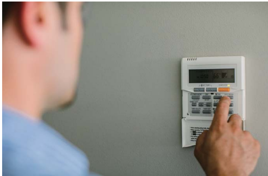
A technician programs a thermostat for one of the home's Halcyon mini-split units.
