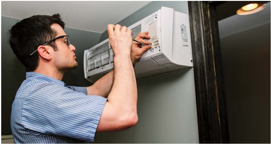
7,000 BTUH wall-hung evaporators were used in the upstairs bedrooms of the new in-law suite.
