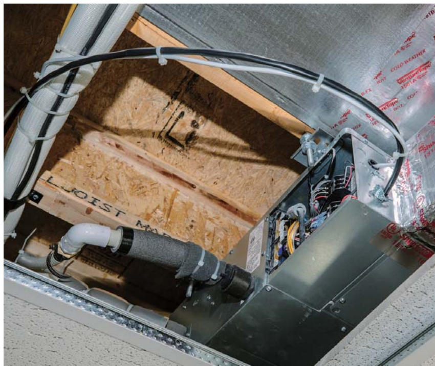
High Efficiency Solutions used slim-duct units above the basement’s drop ceiling to remain above the beam.
