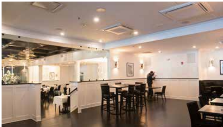
The main dining area at the restaurant features two large, circular flow ceiling cassette units.
