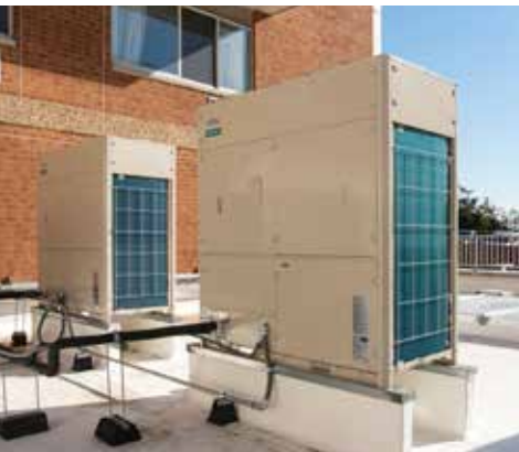
The two, 14-ton Airstage VU-V systems at 160 Prospect Avenue serve a gym and a high-end restaurant.
