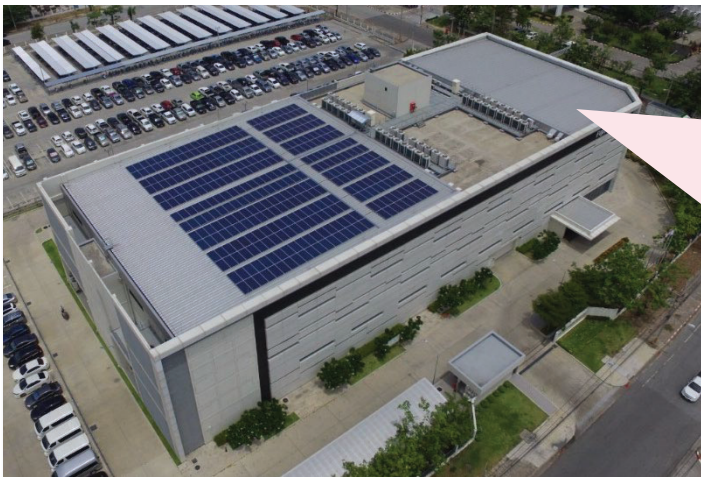
Solar panel newly installed on the roof of FUJITSU GENERAL ENGINEERING (THAILAND) CO.,LTD.
