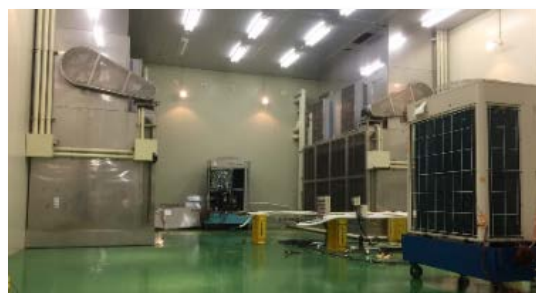
Air conditioner evaluation test room at the head office
