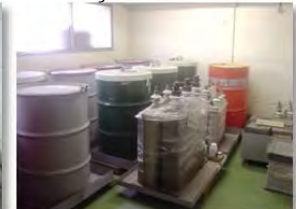
Polychlorinated biphenyl inside the storage of at head office
