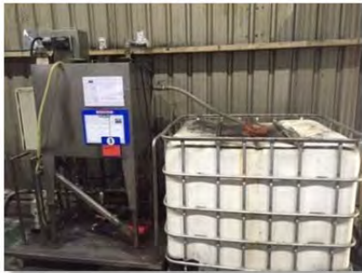
Oil-water separation equipment of FGA
