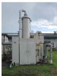
Groundwater purification facility (Aomori Business Office)
