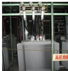
High efficiency transformer introduced at the head office
